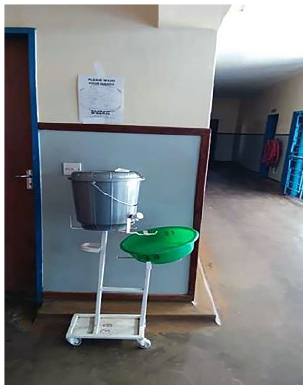
FIGURE 7 Newly purchased washing facilities in situ
